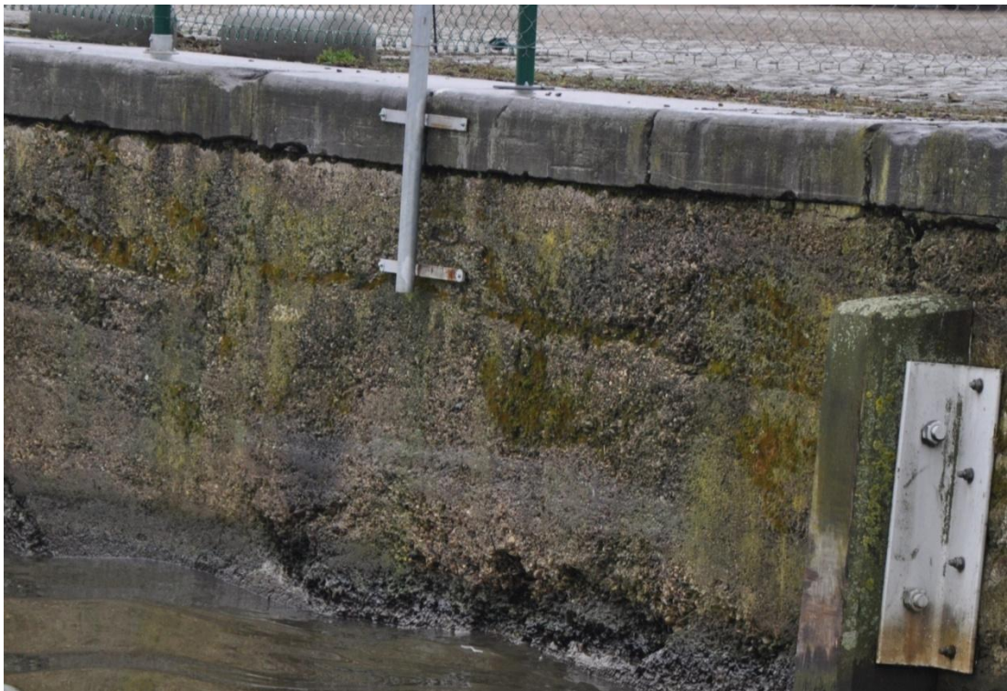
Figure 19: Visual inspection quay wall Biestebroeck Dock – erosion between granite and concrete (source: Technum)
