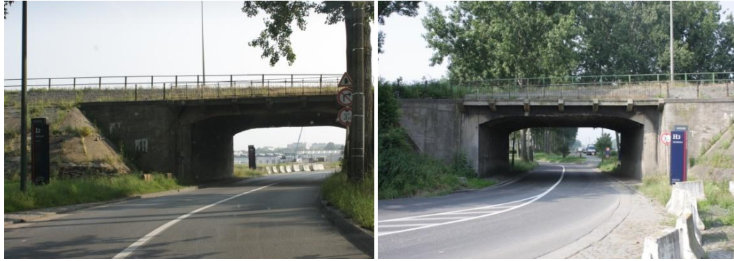
Figure 63: Current configuration of Digue du Canal where it passes under Petite Île bridge (source: Technum)
