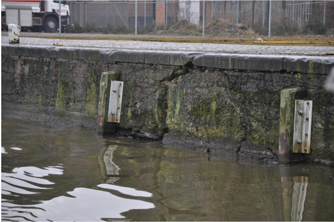
Figure 16: Visual inspection quay wall Biestebroeck Dock – crack in concrete near 20H (source: Technum)
