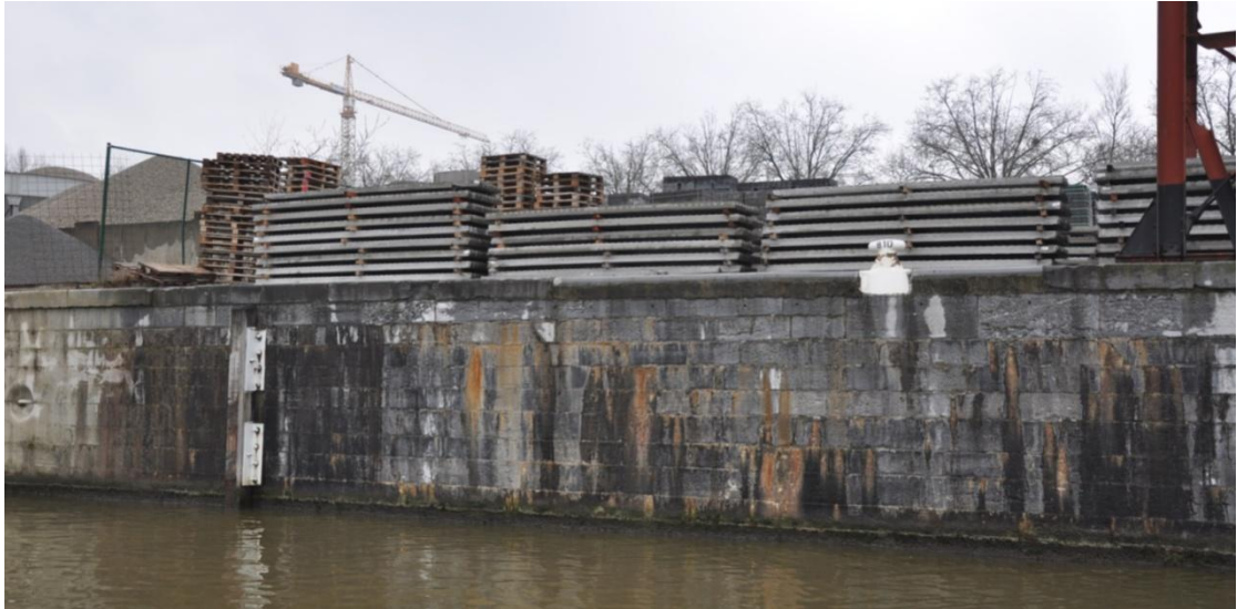
Figure 21: Visual inspection quay wall Vergote Dock – void in granite covering block (source: Technum)
