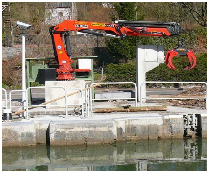
Figure 50: Hydraulic crane on a concrete baseplate built into the quay
