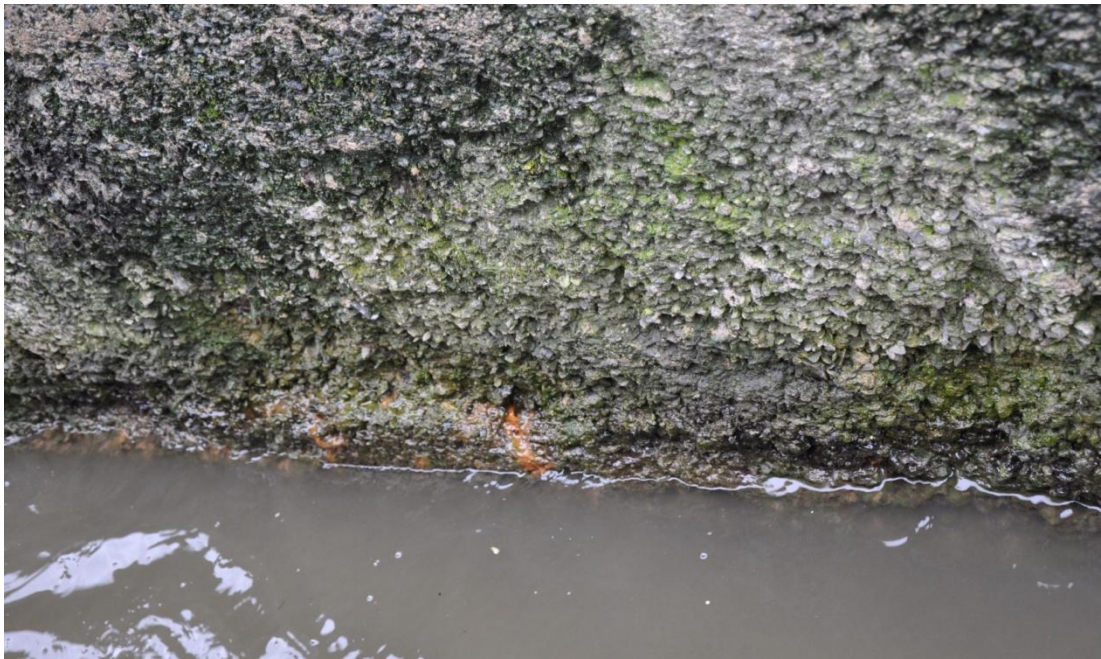
Figure 15: Visual inspection quay wall Biestebroeck Dock – concrete erosion (source: Technum)
