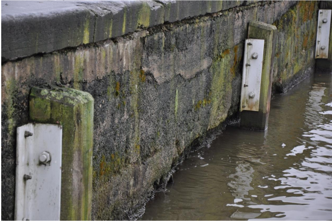
Figure 18: Visual inspection quay wall Biestebroeck Dock – void between concrete structure and fender (source: Technum)
