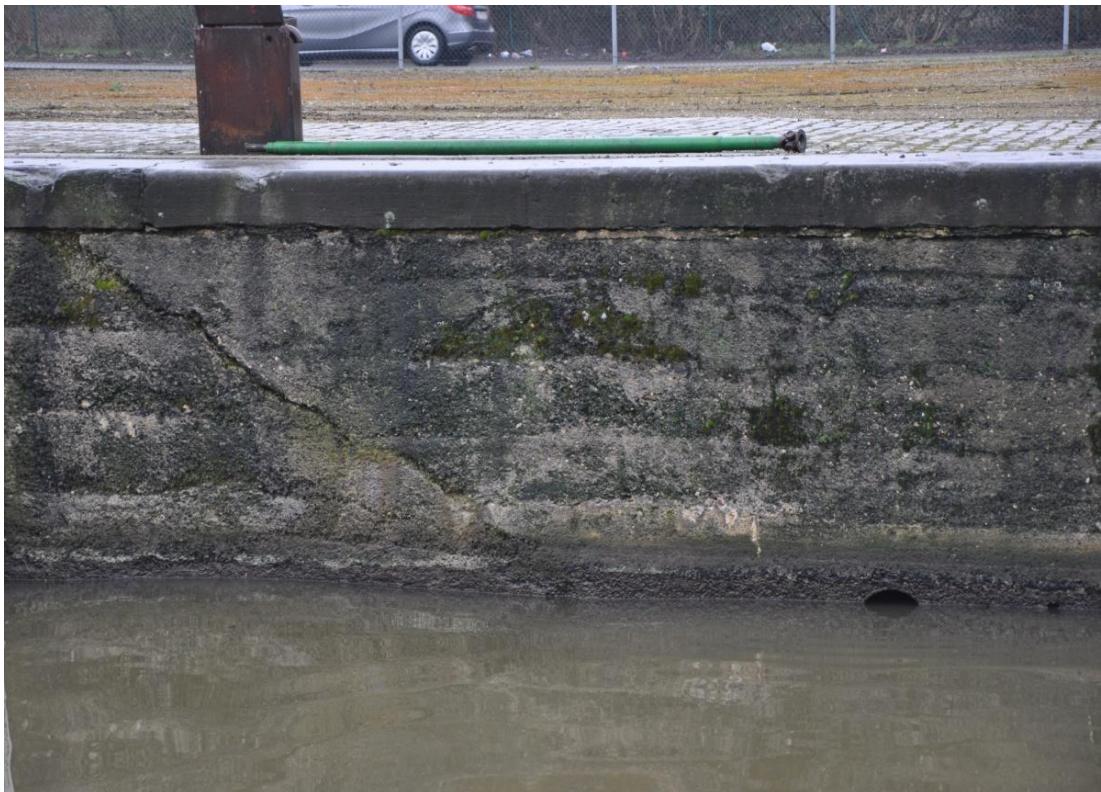
Figure 17: Visual inspection quay wall Biestebroeck Dock – crack and tube in concrete near 20H (source: Technum)
